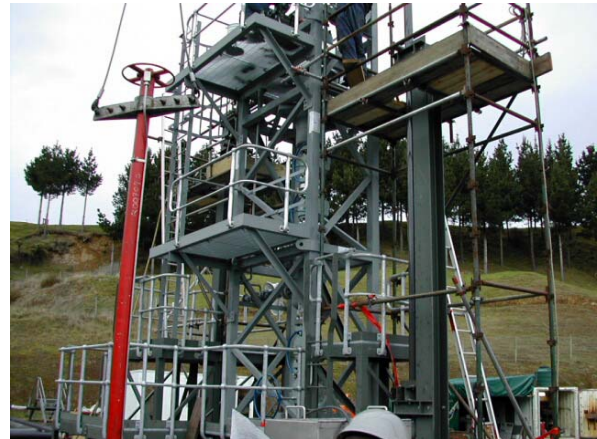
Fig. 8 – Shell Mangahewa 5,000 psi WDC System
